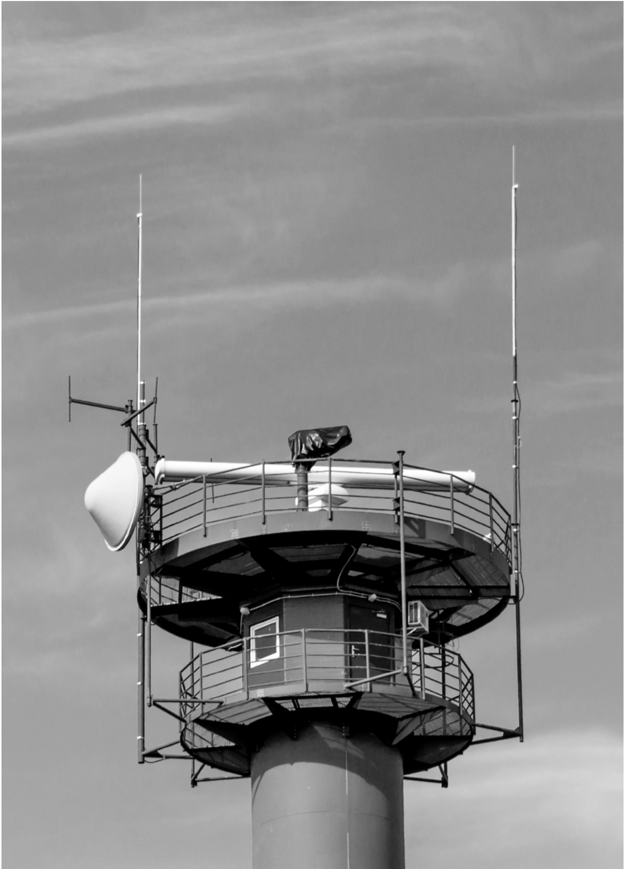
Baltic coastal radar system for maritime traffic monitoring
